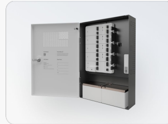
Door access control
